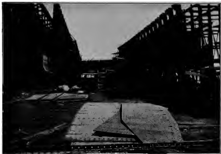
SCENE IN CONSTRUCTION OF STEEL FREIGHTER DANIEL J. MORRELL ABOUT FORTY DAYS AFTER LAYING OF FIRST KEEL PLATE
